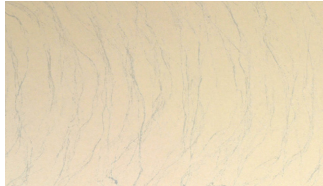
COVERAGE TOO LIGHT
